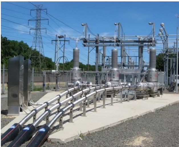
Figure 20. AMSC 3-phase AC HTS distribution line emerging from the ground to transition to conventional power lines (Courtesy of AMSC)
