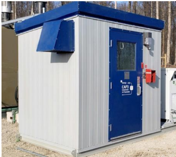
Figure 18. Qnergy CAP field installation
