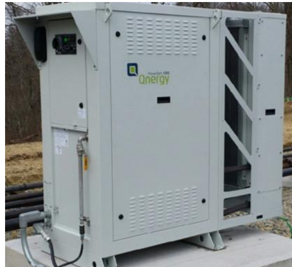
Figure 19. Qnergy PowerGen field installation
