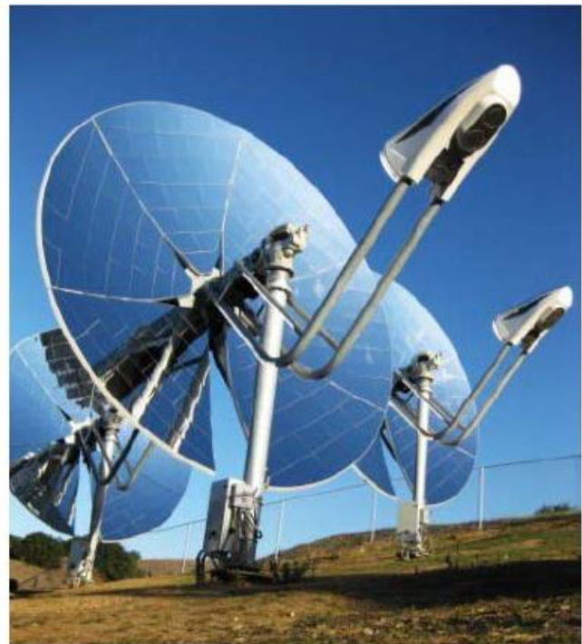
Figure 5. Example of an Infinia dish Stirling installation on uneven ground
